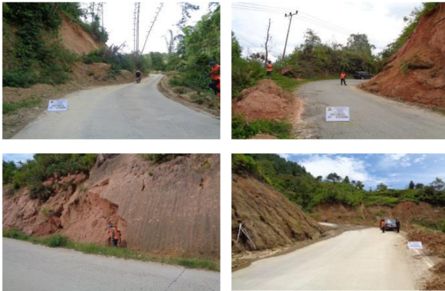
Figure 3. Several landslide spots in the road were observed during the field survey.
